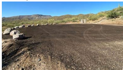
The Town of Cave Creek Public Works crew recently established a helicopter landing site for emergency incidents in the Spur Cross Conservation Area, ensuring safer and faster rescues. (Town of Cave Creek/Submitted)
