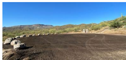
The establishment of a dedicated helicopter landing site will significantly bolster emergency response capabilities in the area.
